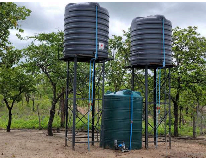
Water Infrastructure: A solar-powered borehole with a 5,000-liter storage capacity
